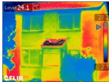
Thermal image of front elevation before refurbishment shows excessive heat loss through the walls and windows.
